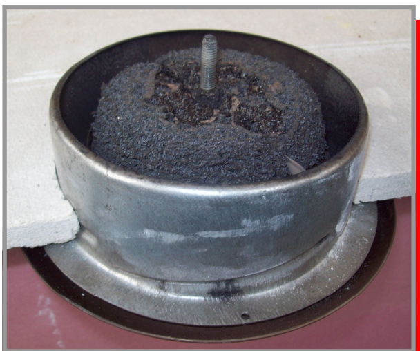
MANROSE Fire Air Valve sealed after a fire
